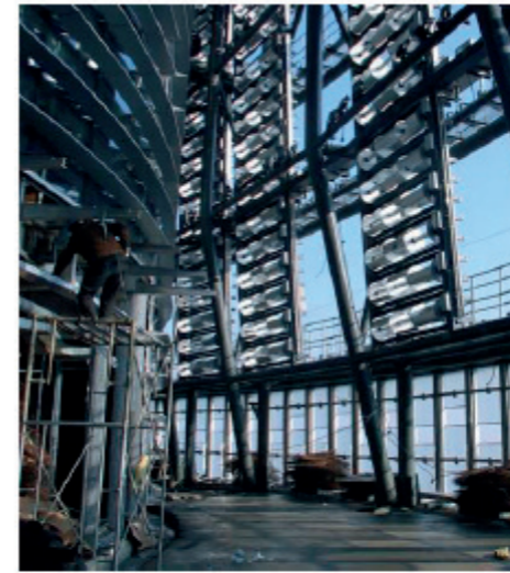
270 Horizontally oriented wind turbines (installed on 122F, 123F and 124F)
